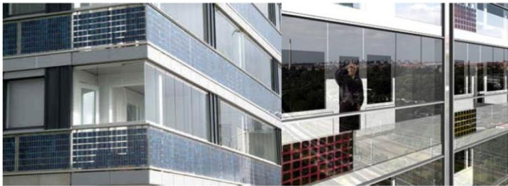
Fig. 3.B.30: spandrels and parapet solutions. Left: Housing Estate, Ekovikki, Finland, Oy Reijo Jallinoja: semi-transparent PV modules with two-paned glazing in parapet areas, Resource: PV NORD. Right: Kollektivhuset, Copenhagen, Denmark, Domus Arkitekter: PV cells were laminated to a single glass, heat transmitted from the cells was used in an innovative way to create thermal comfort during spring and autumn, during summer they are ventilated with an optimized shaft behind the cells and a coloured shutter through airgaps in the bottom and top of the glazing of the balcony, Resource: PV NORD.
