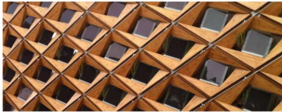
FIGURE 19: A COMPLEX BIPV FACADE IN THE SOLAR DECATHLON "PARA ECO HOUSE" (SOURCE: C. POLO, SUPSI)
